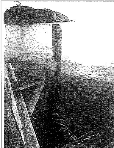
Plate 3: the natural erosion of the hardwood timber piles, embarkation steps and wharf structure is visible here and appears fragile in the face of impacts. One of the proposed piles would be installed on the outside of the pile seen in this photograph (refer engineers plan in Plate 7)
