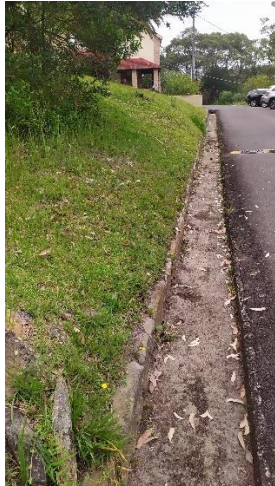
Clear stormwater drain outside S1
