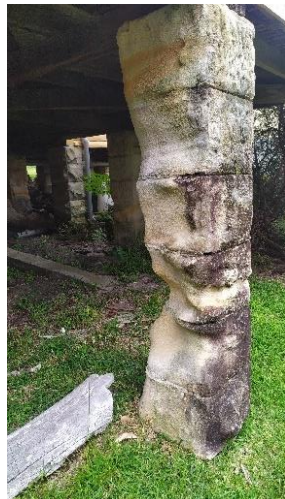
Sandstone pillar in poor condition P1
