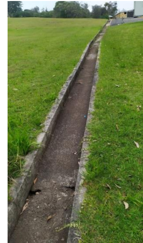
Clear stormwater drain -P13
