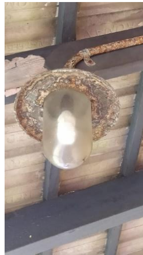
Light fixture with rust P11
