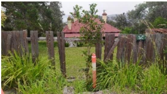
Fencing behind S10 in poor condition
