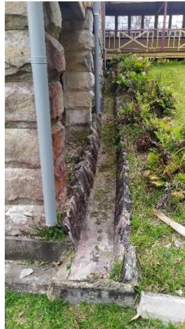
Cleared building drain-P7
